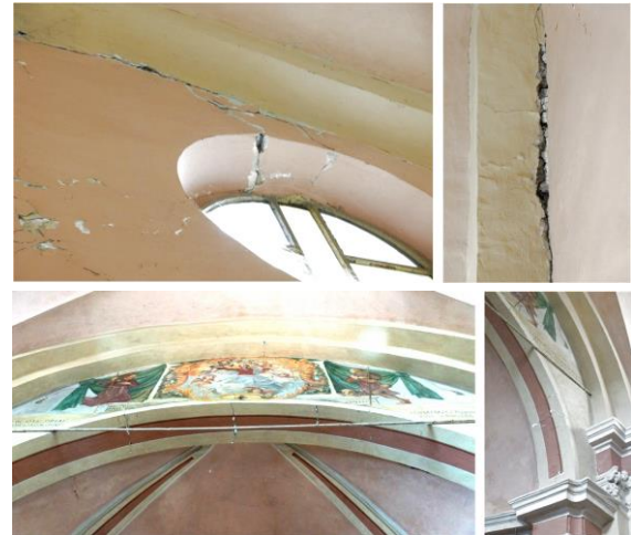
Figure 3. Crack pattern on the masonry structure of San Prospero church after the 2013 earthquake: on the façade (upper); on the intrados of the triumphal arch (lower).
